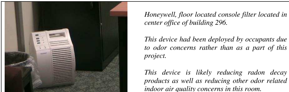
Figure 20: Air Purifier Located in Office of Building 296
